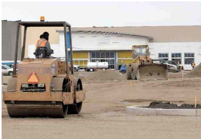
Construction continues on the Grasslands shopping complex in Harbour Landing. Photograph by: Roy Antal, Leader-Post, The Leader-Post
