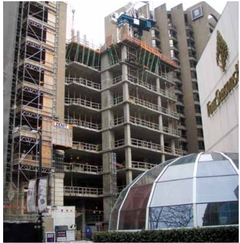
Delta Group's mixed-use Hotel Georgia development (669 Howe Street) is now built up to the twelfth floor. The 71,500-sf office component is slated for completion in fall 2010.
