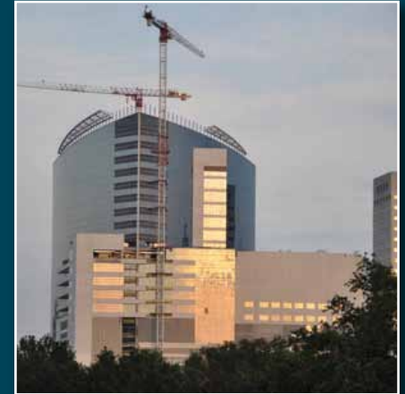
Two construction cranes in the Texas Medical Center provide a sampling of the 26 new projects either under construction or slated for construction prior to 2014.
