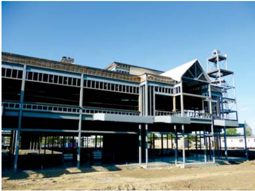
Construction of Gateway Village (30,000 sq. ft.) is underway in the South Side District
