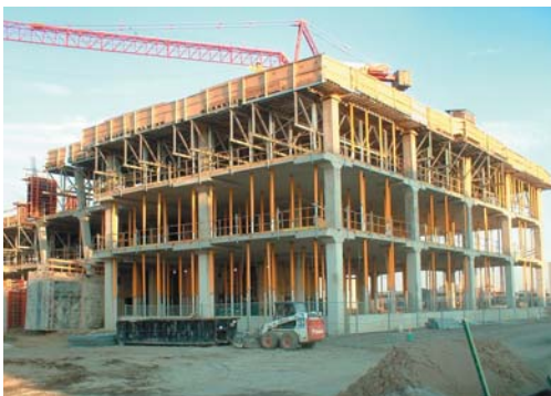
Currently under construction by Redcliff Realty Advisors: 106,866 sq.ft. of office space at 5750 Explorer Drive, Mississauga.
